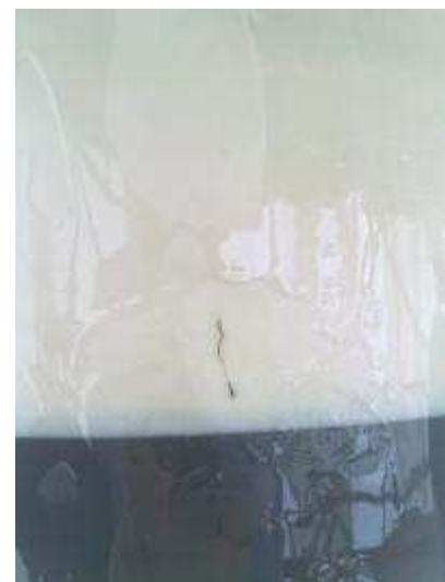
Figure 27 – Treeing traces on the cone of a OTC 500kV external termination.
