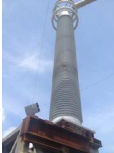
Figure 25 – Directional search of the defect.
