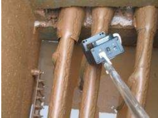
Figure 22 – Localization of the faulty joint in medium-voltage
