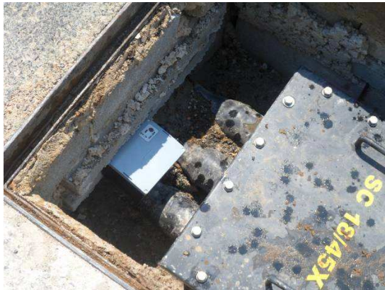
Figure 15 – Online measurement on coax cables coming from the joints.
