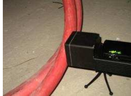
Figure 23 – Localization of the fault on cable - MV
