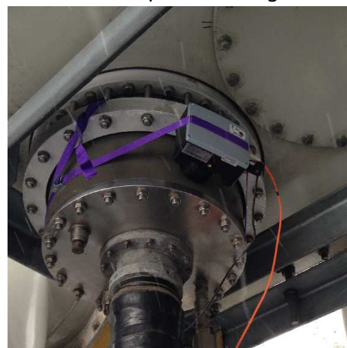
Figure 14 –Measure on a GIS termination.
