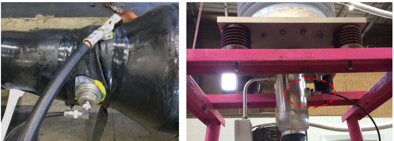
Figure 4 The HFPD sensor as mounted close to joint D (location S_3 , photo left) and close to termination A (location S_1 , photo right).
